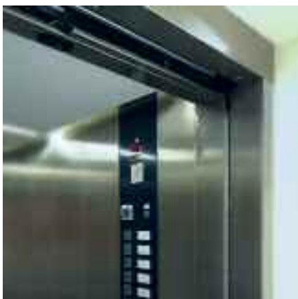
e.g. control of lifts
